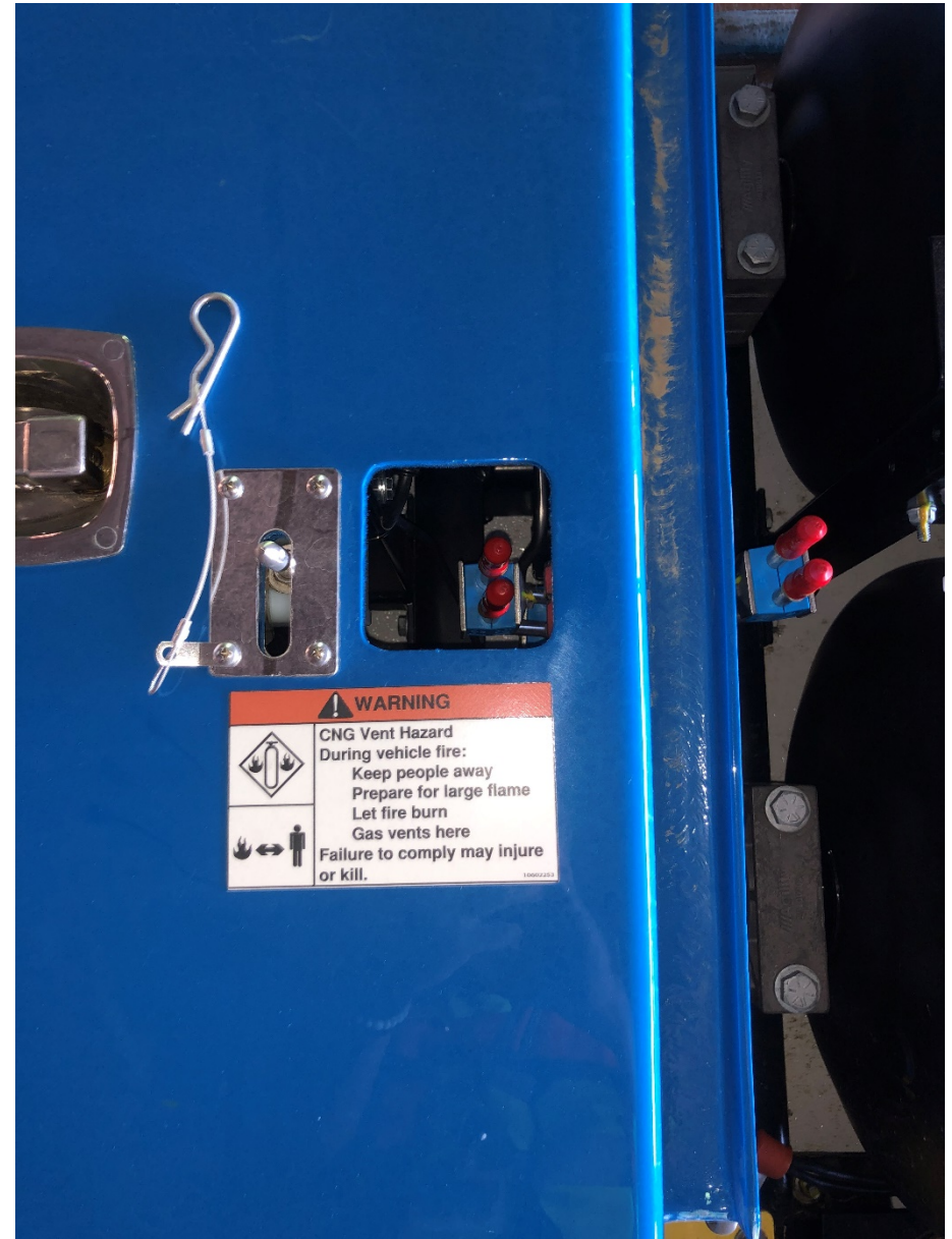
12. PRD vent line outlets (with red cap) on Gillig CNG bus.
