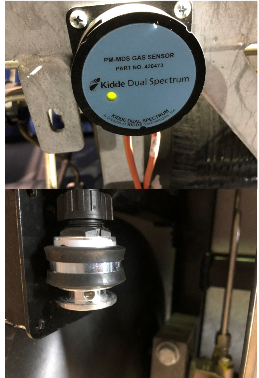
10. Top: Kidde Dual Spectrum gas sensor attached to New Flyer CNG fuel tank compartment. Bottom: Amerex gas sensor attached to Gillig CNG fuel tank compartment.
