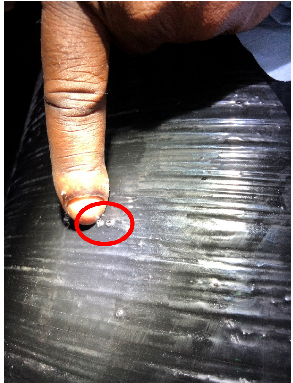
8. Inspector points to an anomaly on the surface of the tank; i.e. two (2) resin bubbles. Resin bubbles can occur during the manufacture of the tank and are not considered a structural defect.
