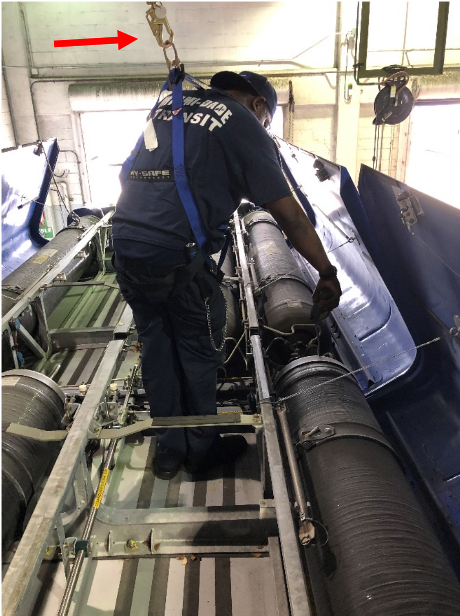
3. Inspector using a portable leak detector to wand in and around valves, gauges, and PRD with a portable leak detector. Red arrow shows inspector in safety harness attached to tether line.
